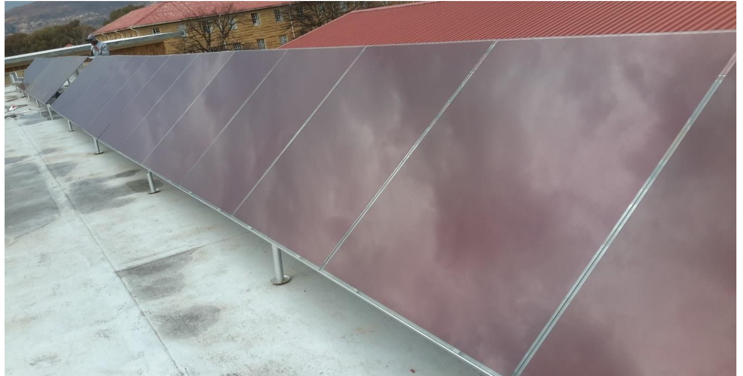
NUL Library Grid Connected 2.4 kWp Solar PV Plant
